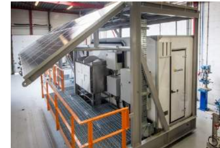
Skid mounted GRP battery shelter
