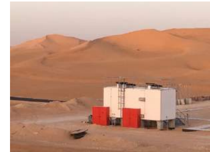
Passive shelter with Fire fighting protection
