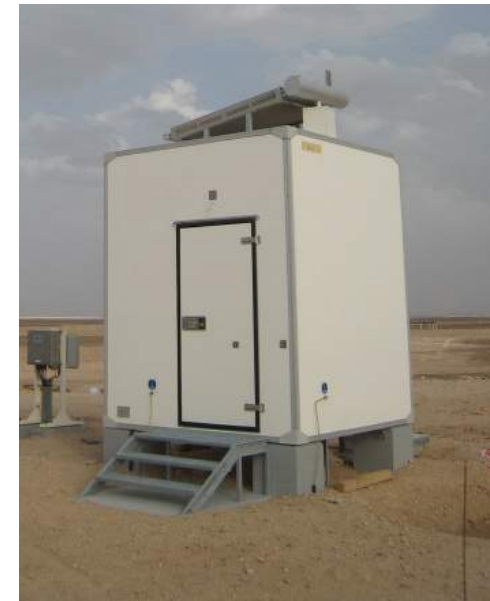
Passive cooled Shelter
