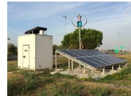
PCS with solar and wind turbine
