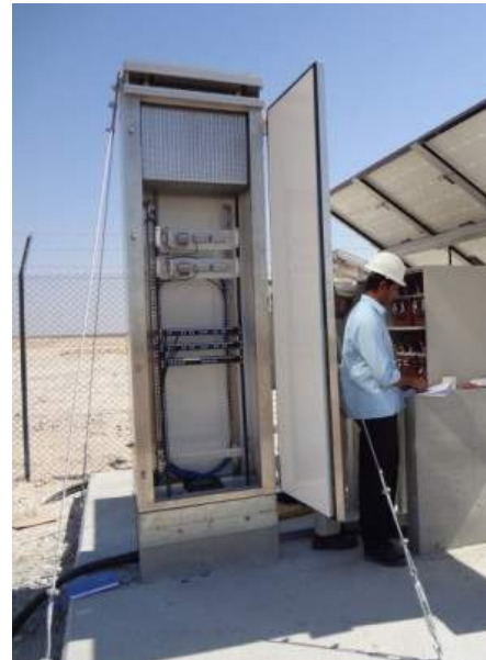
Passive cooled cabinet
